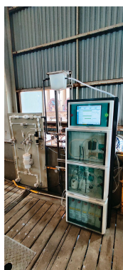
Figure 2. 2060 TI Process Analyzer with preconditioning panel in a zinc refining plant.
